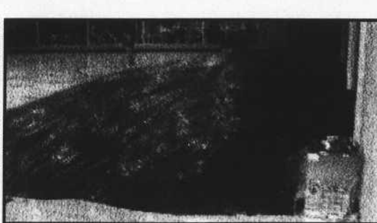
Photo by Chris Dunn The recent cold weather is being blamed for the broken pipe that has closed part of Spaulding Gym.
